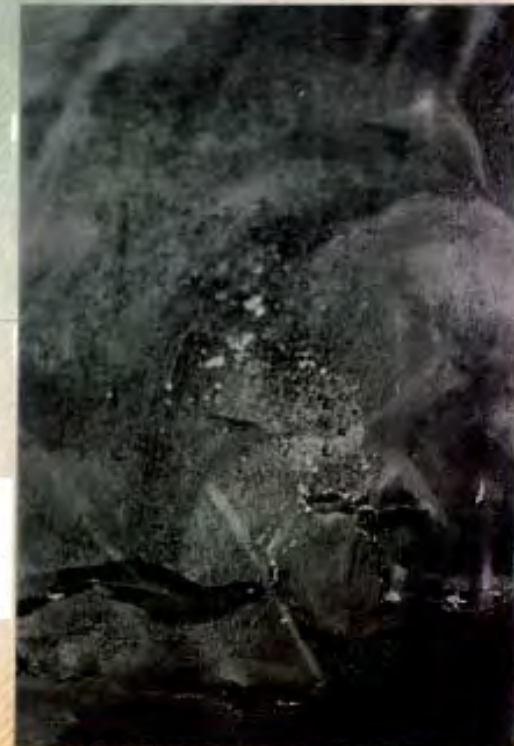
THE ONLY FIRE DAMAGED AREA BEHIND THE CORNER WALL 3
